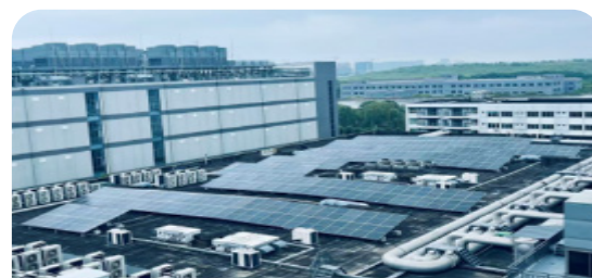
Photovoltaic on the roof of data center
